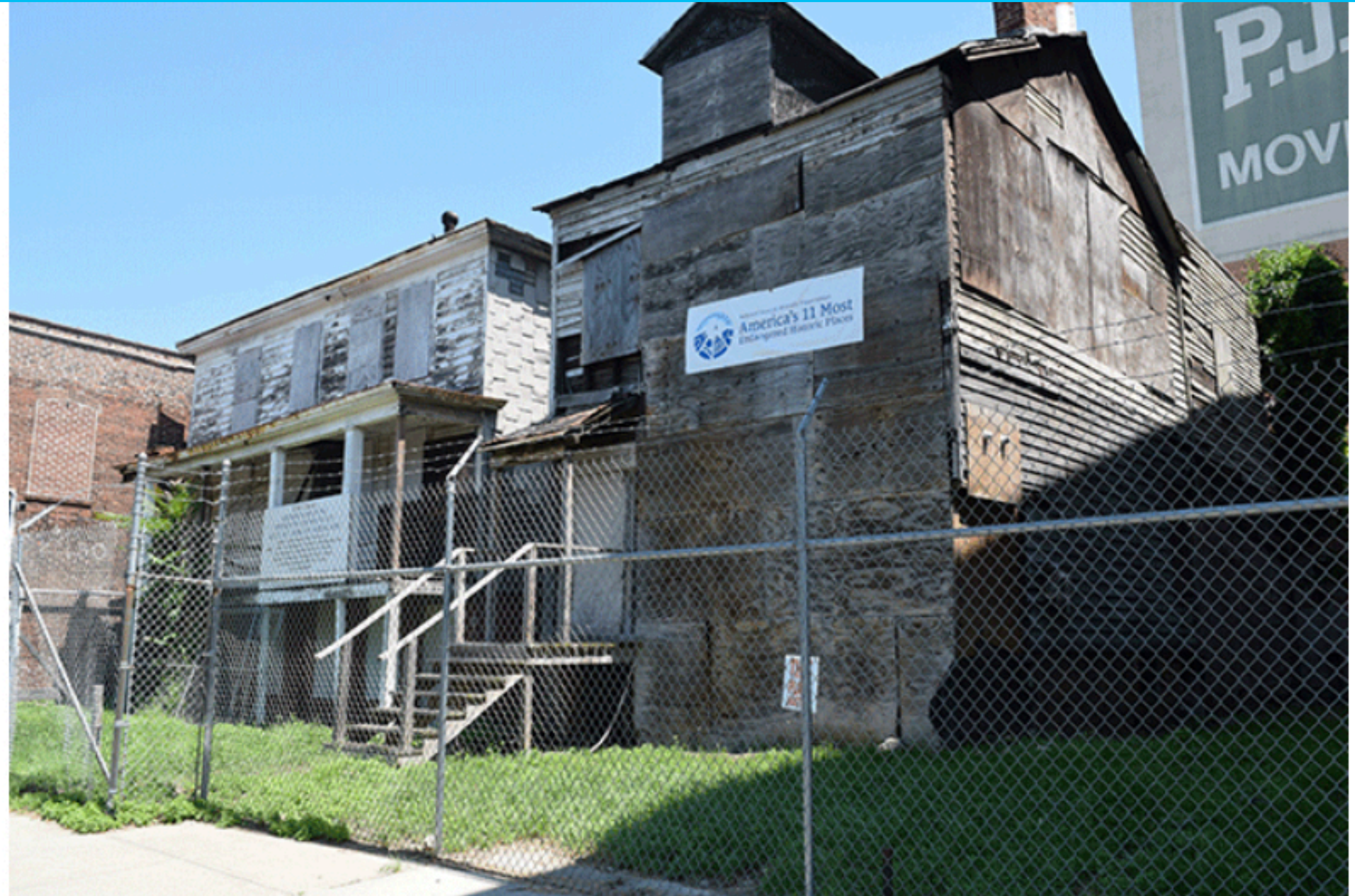
The Mary and Eliza Freeman Houses on Main Street in Bridgeport's South End. Photo by Phil Hall.
